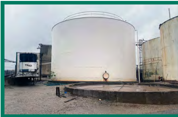
TANK #2 734,000 GALLON CAPACITY 1 1/2" WALL THICKNESS
