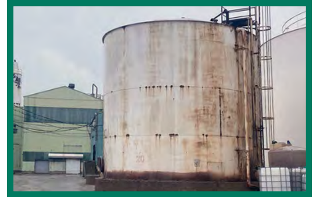
TANK #3 142,537 GALLON CAPACITY 3/4" WALL THICKNESS
