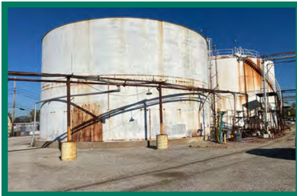
TANK #1 676,776 GALLON CAPACITY 1 1/8TH" WALL THICKNESS
